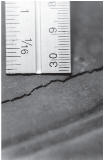
Figure 8. External side of a transverse crack.
