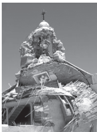
Figure 1. Bell tower in Northern Chile collapsed by an earthquake in 2005.
